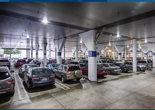
New LED lighting in the mall's parking garage.
