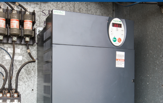
Close-up view of one of the new VFDs.
