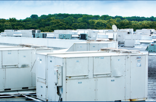
VFDs were installed in these rooftop HVAC units.
